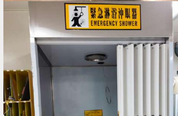
▲ Emergency body and eyewash station
